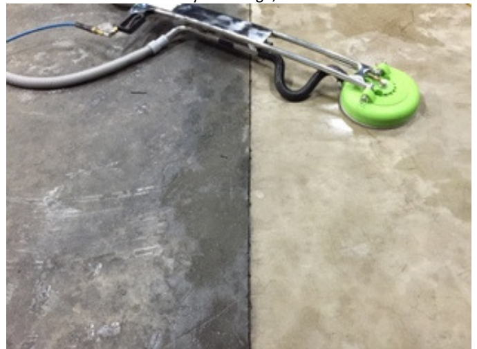
Before/After Photo of Concrete Floor at Meat Processing Facility in Chicago, IL
